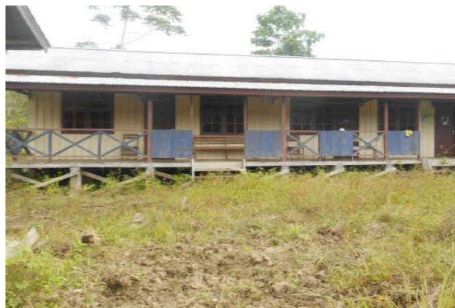
Picture 5: The condition of the auxiliary health center (PUSTU) in Kwarja village, Jayapura district. Photo: Archives of JPIC Franciscan Papua
