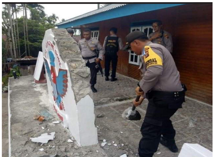
Demolition of KNB Secretariat by the Police Source: KNPB
